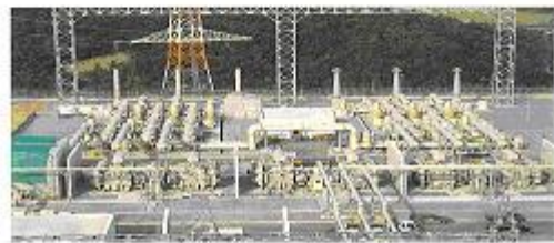
765 kV 2000 MVA Transformer bank in KEPCO substation, Korea
