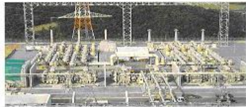
765 kV 2000 MVA Transformer bank in KEPCO substation, Korea
