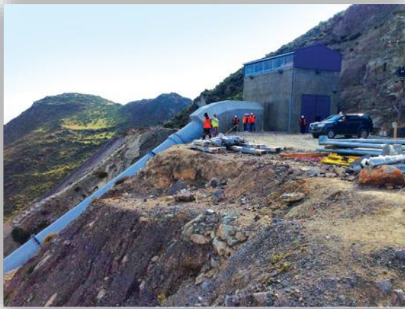
The penstock operates under a maximum design head of 800 m. Photo courtesy: Stantec
